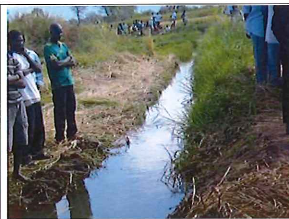
The community helped to construct the subsidiary channels of the irrigation scheme
