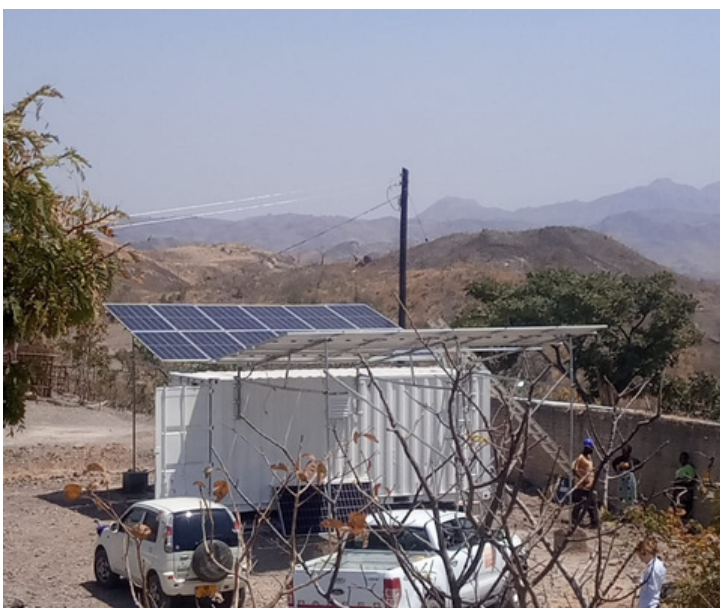
The power generation unit at Kudembe site in Dedza under the EASE project
